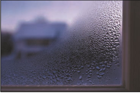
Condensation on the inside of a window-pane
