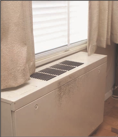
Mold growing on the surface of a unit ventilator.
